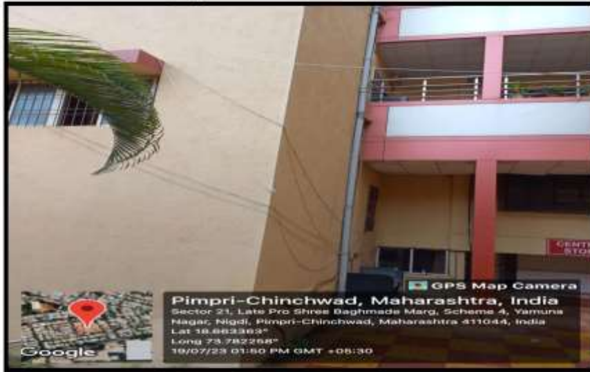
RO Plant water discharge pipeline
