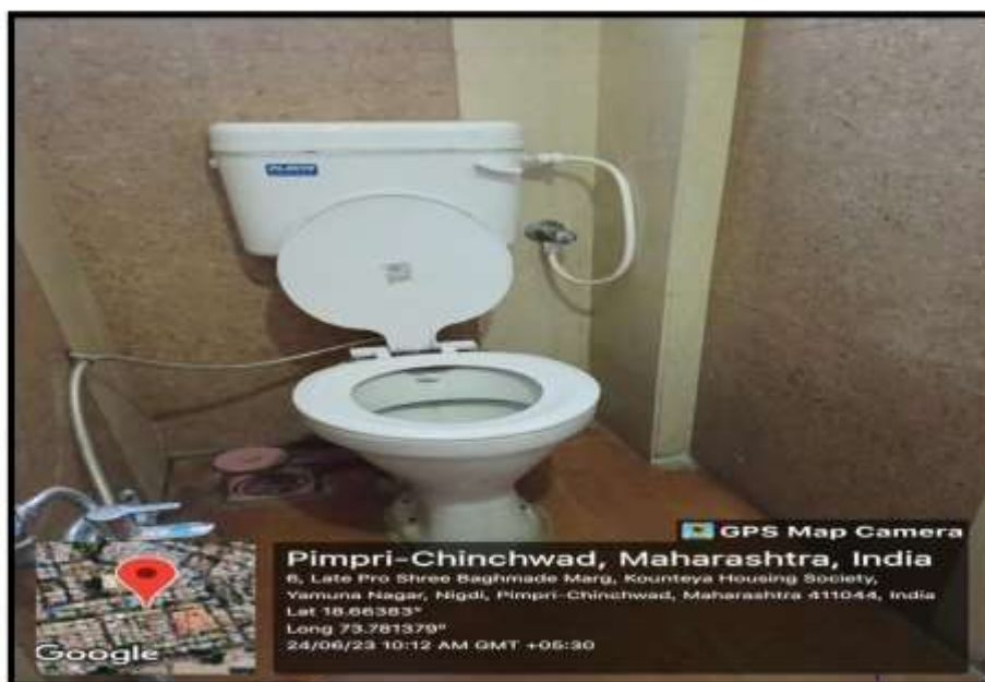
Differently Abled Friendly Restroom
